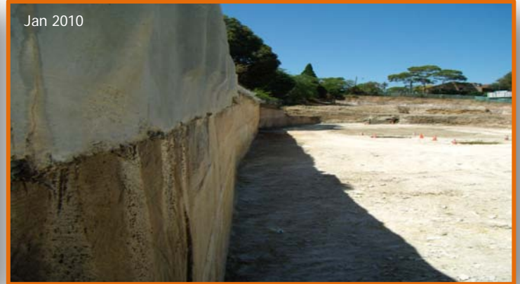
The sandstone rockface was cut with a large diamond tipped cutting wheel that was attached to an excavator
