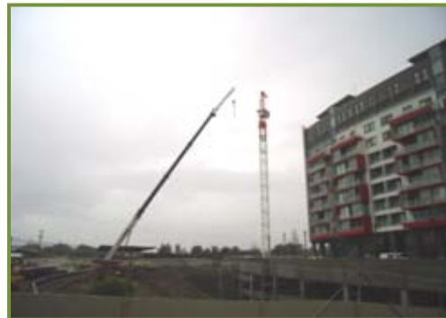
Step 6 Control Cabin & A Frame
